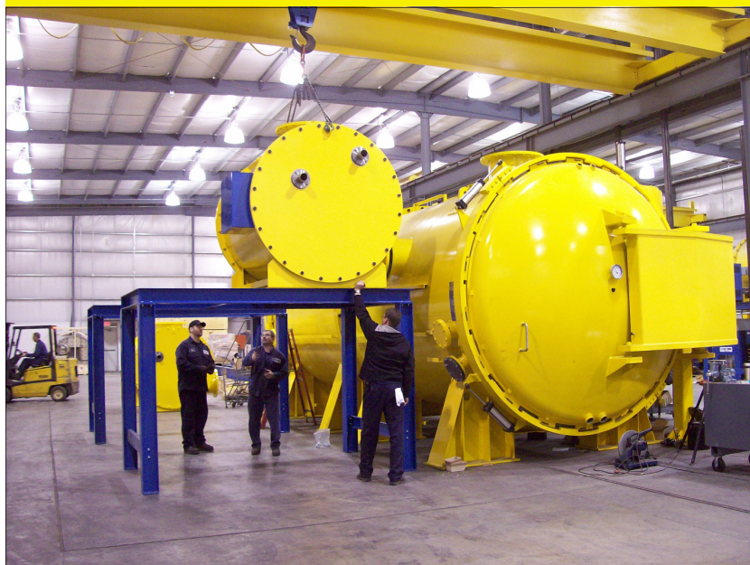
The new 24-foot vacuum furnace being installed at Solar Atmospheres of Western PA
